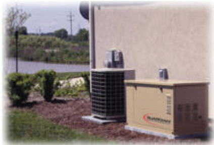
Guardian Emergency Standby Generator
